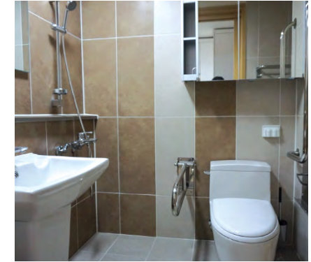
Toilet fitted with grab bars.
