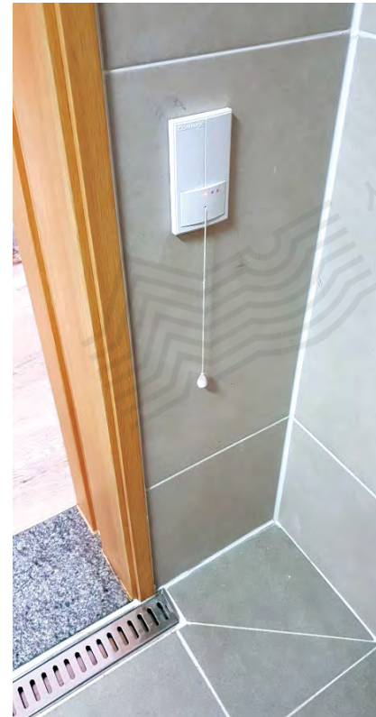
Emergency alarm installed in the bathroom.
